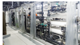
Reverse osmosis (RO) membrane treatment equipment in the water treatment facility at the Mie Recycle Center to recycle water resources
